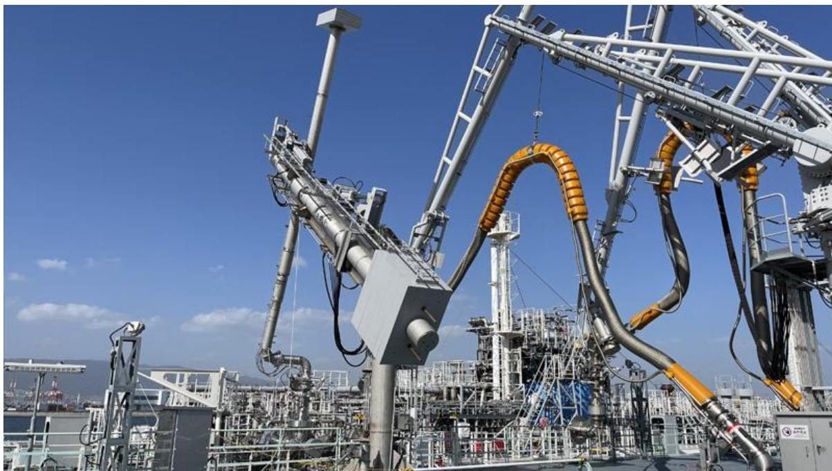
Figure 22: A ship-to-shore rigid Loading Arm System (LAS) installed in the hydrogen terminal at Port of Kobe, Japan. Credit: HySTRA.
