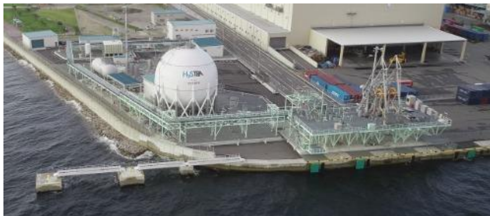
Figure 23: The world's third largest liquid hydrogen tank forms part of an import terminal at Port of Kobe, Japan and can store 178 tonnes 68 (image: HyTouch Kobe).
