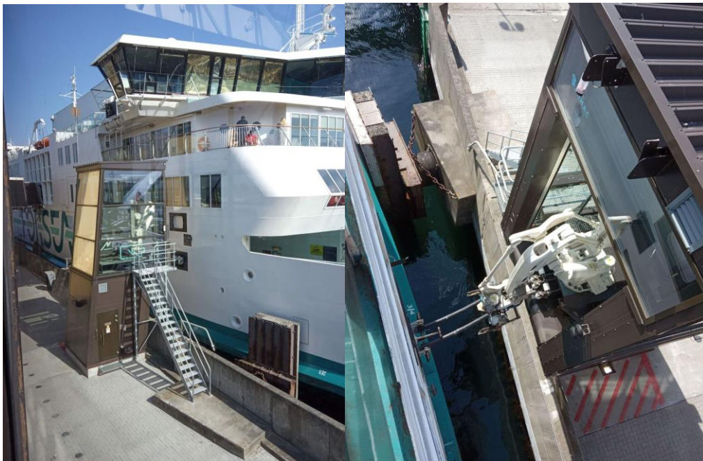
Figure 5: Shoreside 10.5 MW charging connection for Aurora at Helsingborg and Tycho Brahe passenger ferries (images: ZESTAs).
