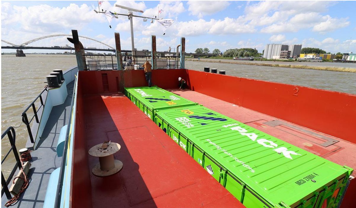
Figure 6: Swappable ESS in 20-foot ISO container operational on inland vessel Alphenaar (image: Zero Emission Services).
