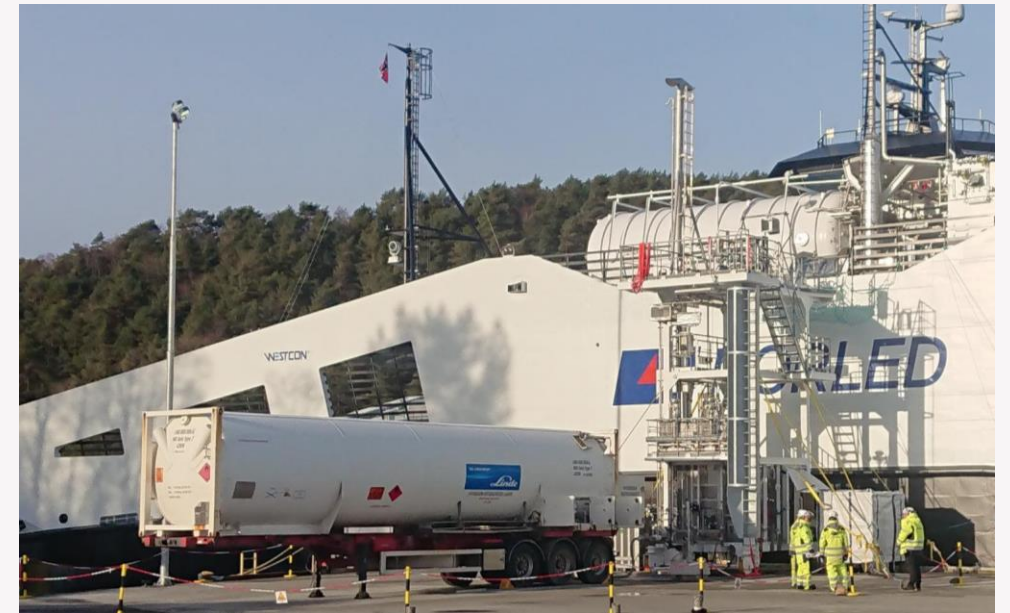
LH 2 bunkering of M/F Hydra using LH 2 transport containers. Method to be scaled for future projects. Picture: Østvik
