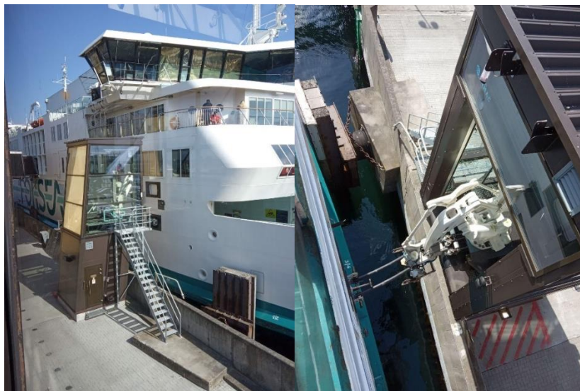
Figure 2: Shoreside fixed 10.5 MW charging connection for Aurora of Helsingborg and Tycho Brahe passenger ferries.
