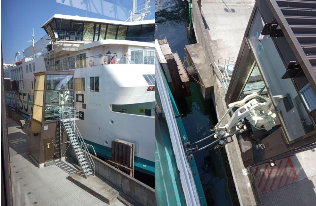
Figure 4: Shoreside 10.5 MW charging connection for Aurora of Helsingborg and Tycho Brahe passenger ferries.
