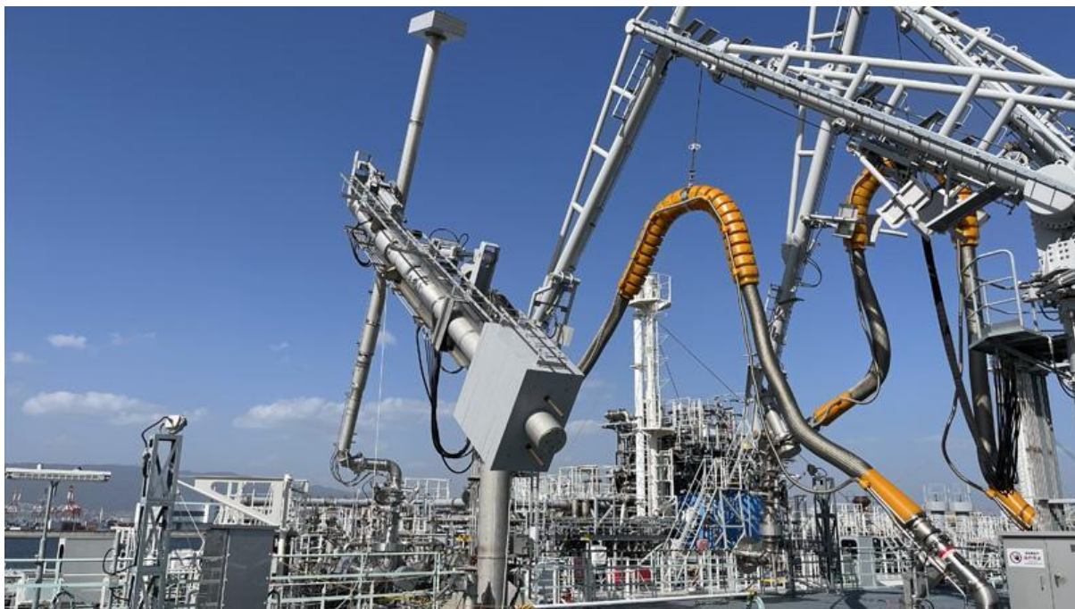
Figure 22: A ship-to-shore rigid Loading Arm System (LAS) installed in the hydrogen terminal at Port of Kobe, Japan. Credit: HySTRA.
