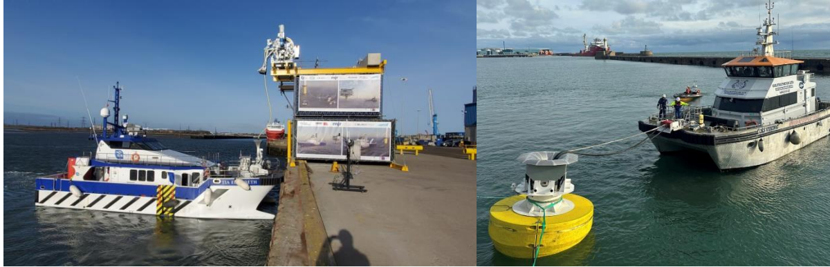
Figure 5: Harbour trials of offshore charging systems. Left: 1.5 MW charging point to be fixed on an offshore structure (image: MJR Power & Automation). Right: floating buoy charging point (image: Jebb Smith Ltd)
