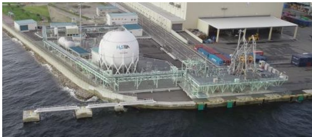
Figure 23: The world's third largest liquid hydrogen tank forms part of an import terminal at Port of Kobe, Japan and can store 178 tonnes 81 (image: HyTouch Kobe).
